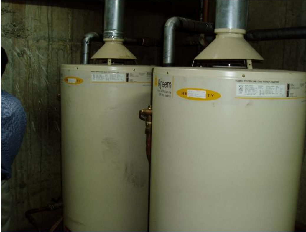
Figure 4 Domestic hot water units
