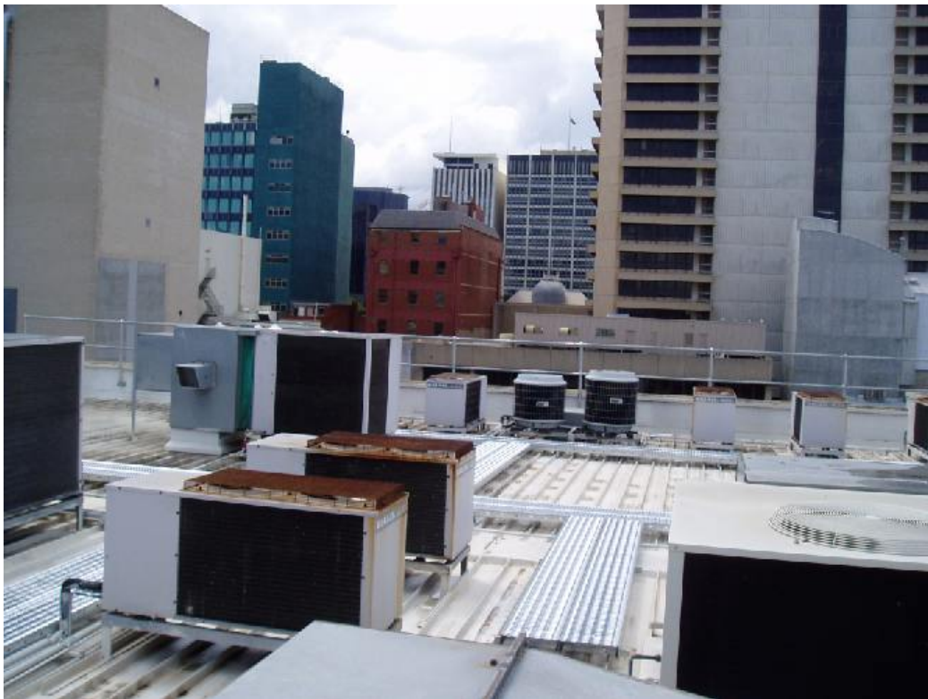
Figure 2 3 rd Floor roof showing some of the air conditioning units
